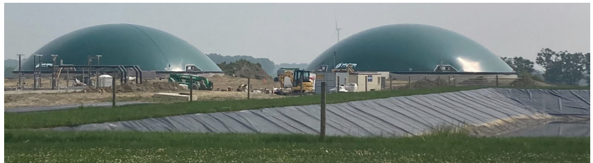
Two digesters are under construction at Lent Hill Dairy Farm in NY.
